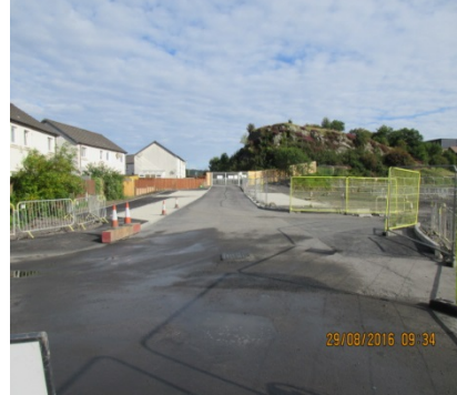
20b New access road and footpath with gates closed during times school in session
