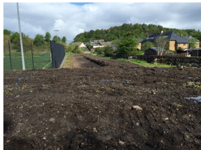
15 Excavation works for the new long/triple jump run up and sand pit
